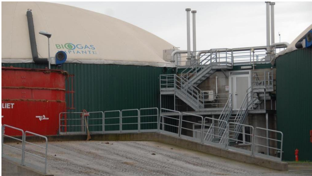
Figure 167: Raised passages in a biogas plant Source: L'Arena.it
