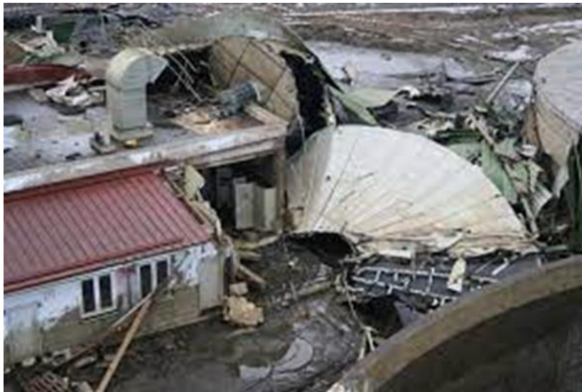
Figure 162: Explosion of a biogas plant Source: Santafocadelfiuli.it
