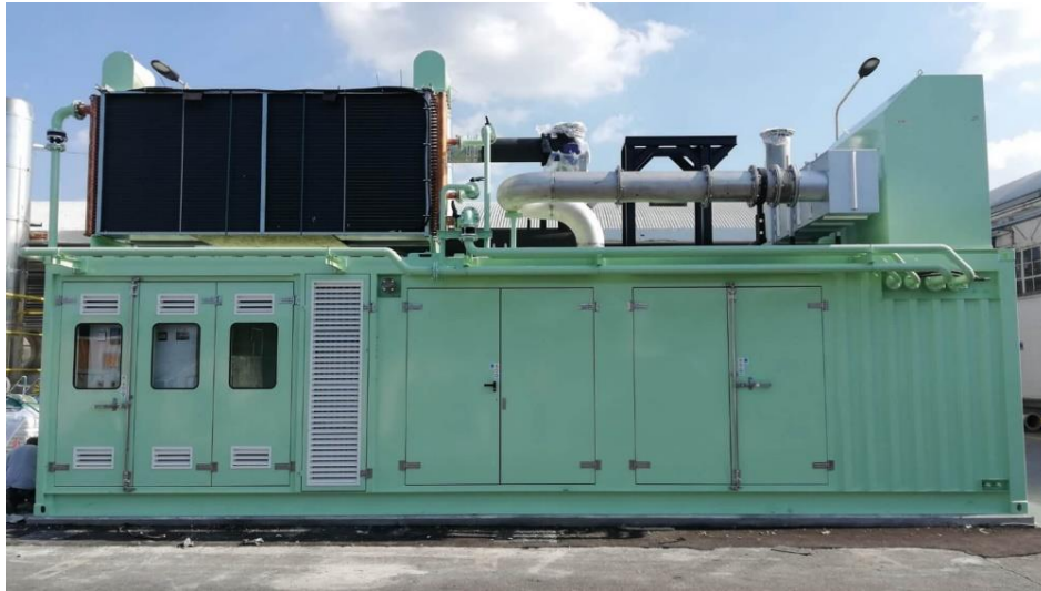
Figure 22: Biogas co-generator Source: Energas
