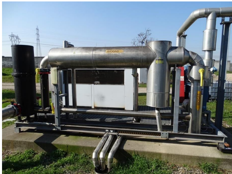
Figure 21: Dehumidification unit Source: Bricchi Alessandro e Ambrogio s.s.
