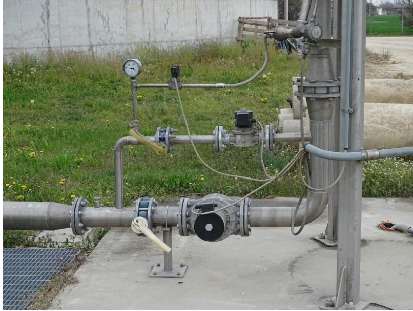
Figure 50: Safety torch solenoid valves Source: Principi di Porcia e Brugnera
