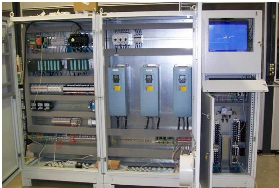
Figure 172: Plant electrical power cabinet Source: Tecnoeffesrl.com
