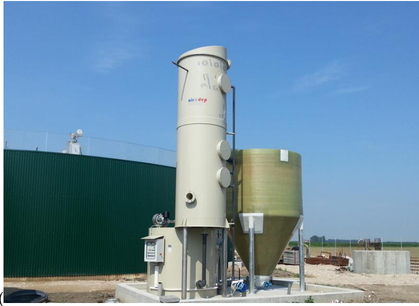
Figure 20: Tower desulphurization Source: Airdep.eu
